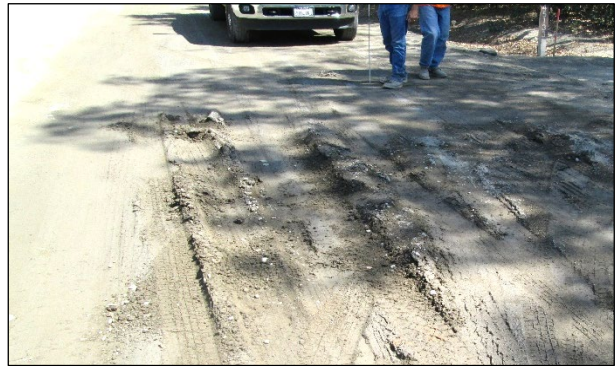
Figure 6.22: Wet area caused by water leaks during tanker change (FDR).
