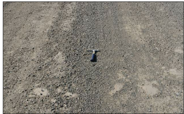
Figure 6.122: Unacceptable surface prior to tack coat application.
