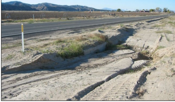
Figure 2.6: Example blocked side drains and culvert.
