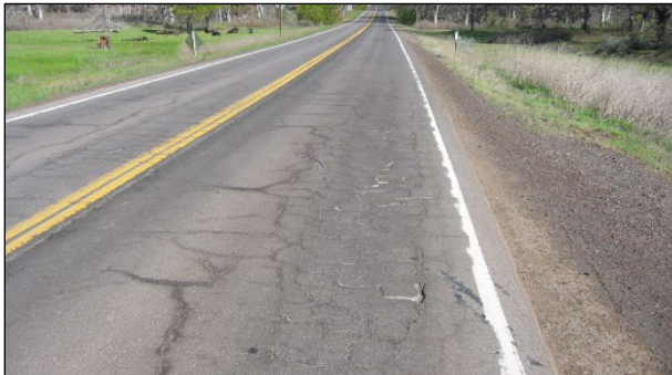
Figure 2.19: Example bottom-up distresses: Fatigue (alligator-B) cracks.
