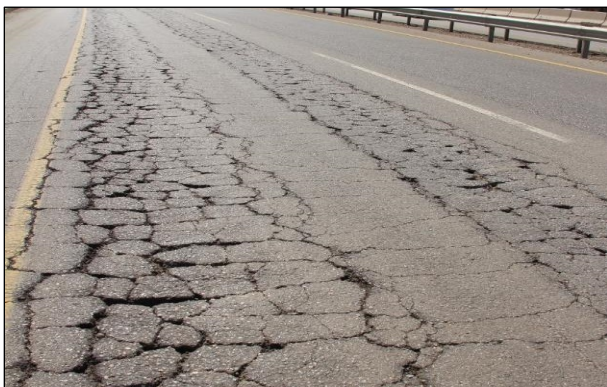
Figure 2.27: Loose blocks in severe alligator-B cracking.
