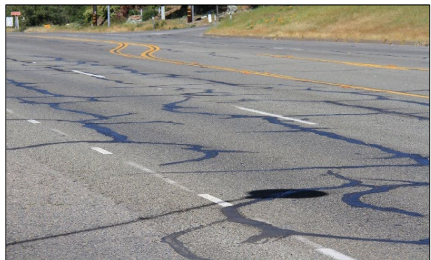
Figure 2.24: Example bottom-up distresses: Sealed reflective cracks.
