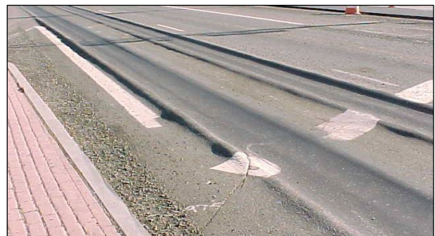
Figure 2.14: Example top-down distresses: Surface ruts during high temperatures.
