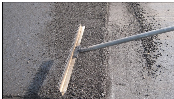
Figure 6.88: Raking to clear material and provide a sight line for the roller operator.
