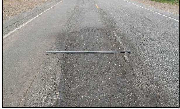
Figure 2.26: Example bottom-up distresses: Ruts associated with subgrade failure (b).
