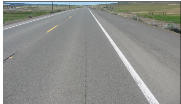
Figure 6.72: Reflected longitudinal crack in area of cement spread overlap (FDR-C).
