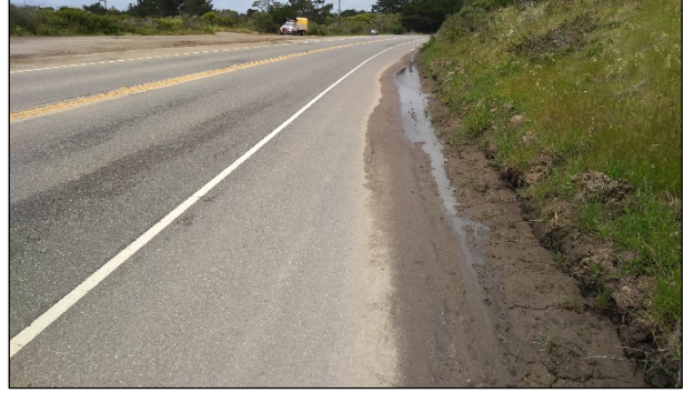
Figure 2.7: Example drainage problem in cut.
