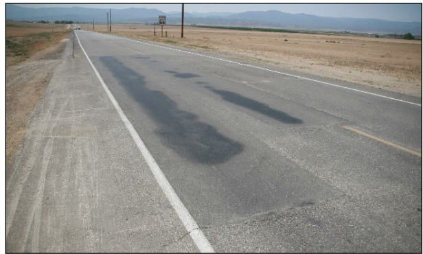
Figure 2.32: Bleeding in wheelpath repairs.
