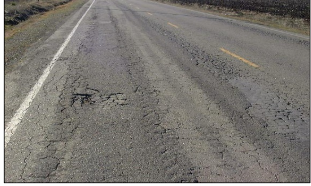
Figure 2.30: Fatigue cracking and potholes in wheelpath repairs.
