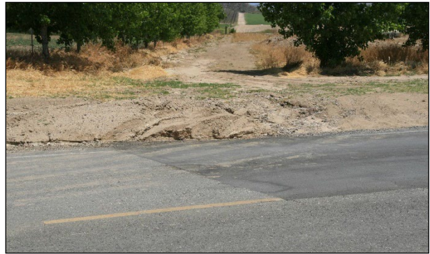
Figure 2.36: Access road drainage problems (note patch).
