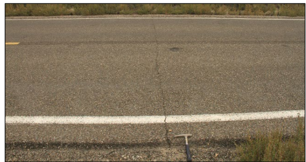
Figure 2.12: Example top-down distresses: Low temperature thermal cracks.
