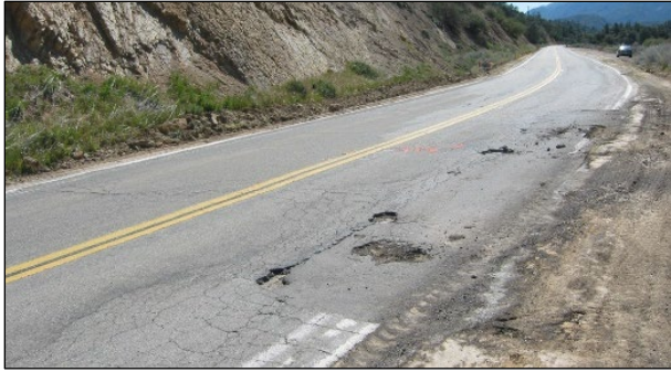
Figure 2.17: Example top-down distresses: Potholes.
