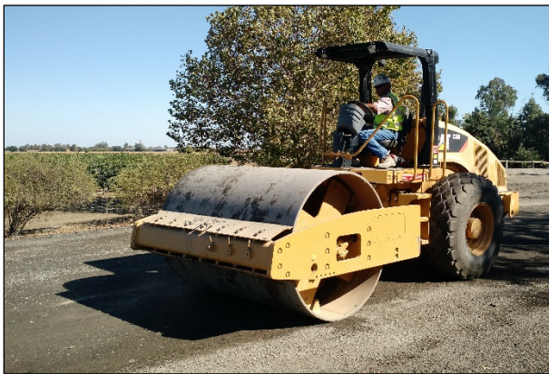
Figure 6.113: Shrinkage crack mitigation (microcracking) on an FDR-C layer.
