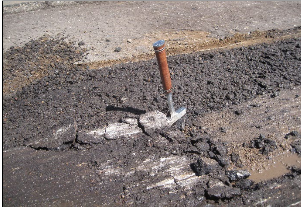
Figure 6.53: Thin, debonded layer on a PDR project.
