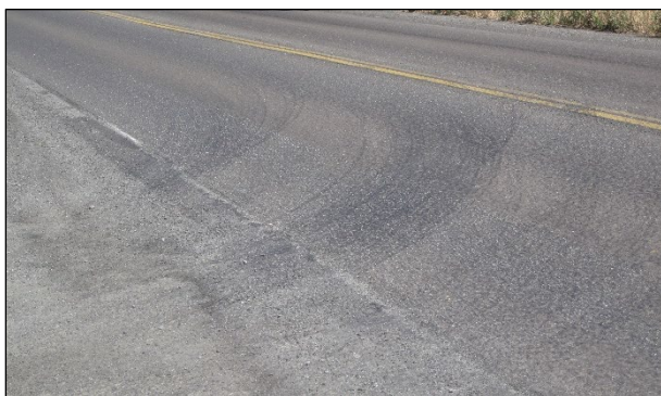
Figure 6.51: Trafficked recycled layer with no raveling/scuffing from turning vehicles (PDR).
