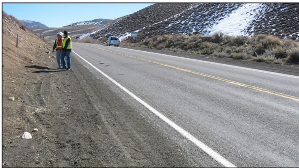
Figure 2.37: Absence of drains below cut slopes.
