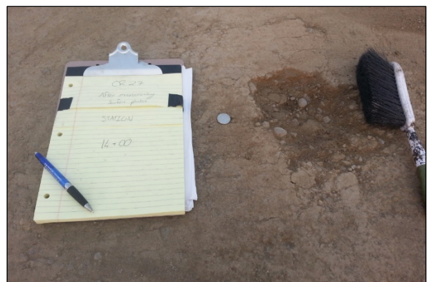
Figure 6.111: Breakup of surface of an FDR-C layer caused by carbonation.
