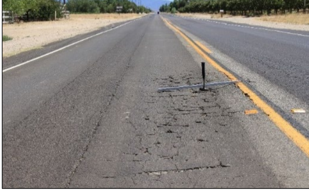
Figure 2.25: Example bottom-up distresses: Ruts associated with subgrade failure (a).
