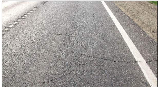
Figure 2.20: Example bottom-up distresses: Block cracks.
