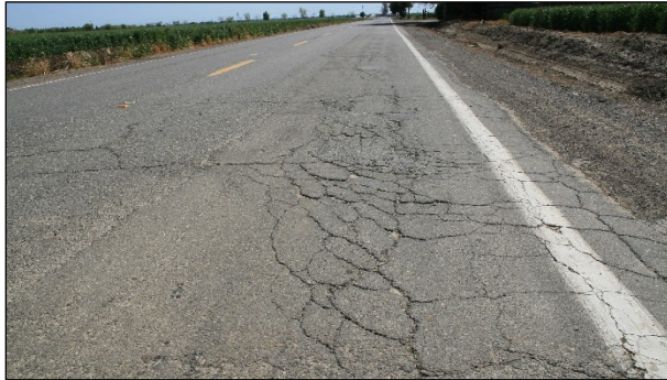
Figure 6.4: Distressed road prior to addition of new layer.
