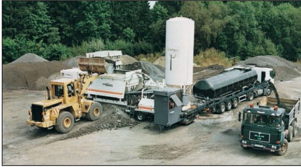
Figure 6.10: Cold central plant.
