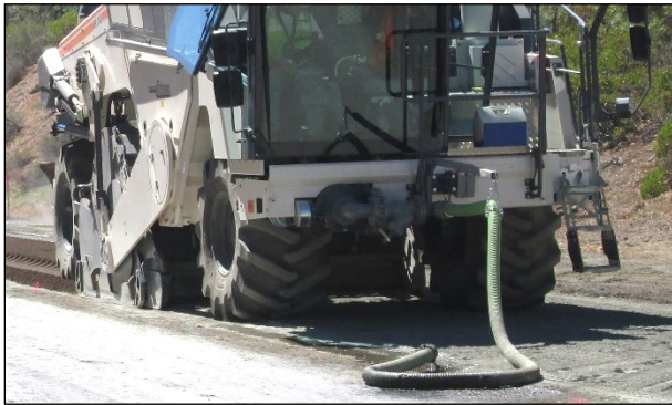
Figure 6.21: Water leak during tanker change (FDR).
