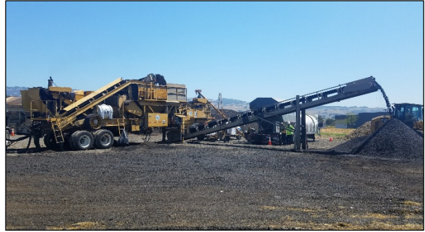
Figure 6.11: Cold central plant using processing unit from a multi-unit recycling train.
