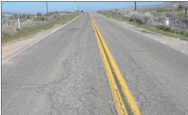
Figure 2.4: Example alligator-B cracking.
