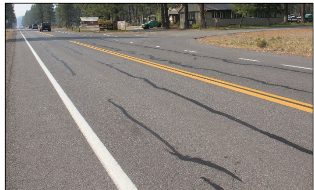
Figure 3.6: Alligator-A cracking on a PDR project.
