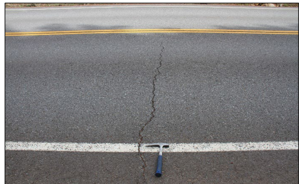
Figure 6.70: Reflected shrinkage crack in area of cement accumulation on an FDR-C project.
