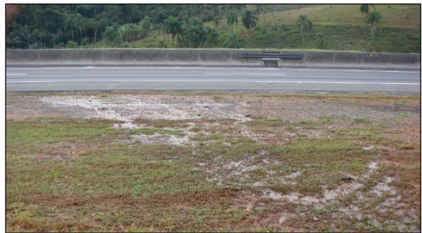
Figure 2.38: Water flowing downslope into the road.
