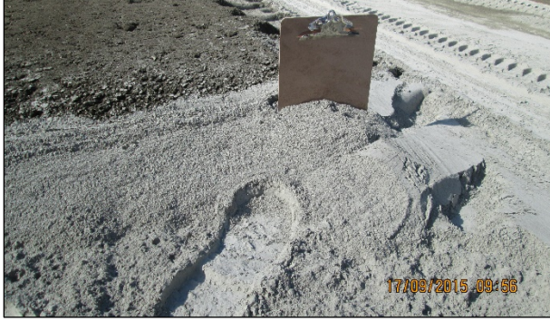
Figure 6.19: Accumulated cement dragged by hose at end of recycling run (FDR-C).
