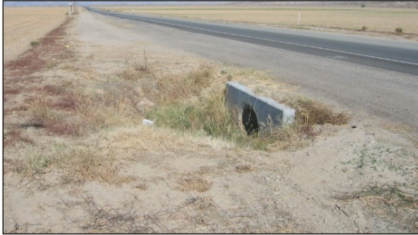
Figure 2.33: Blocked side drain and culvert.
