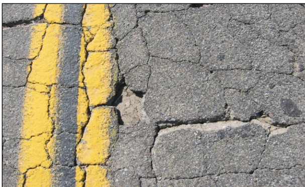
Figure 2.23: Example bottom-up distresses: Unsealed reflective cracks.
