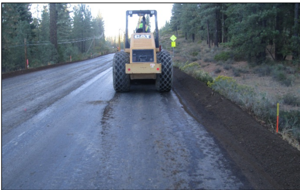
Figure 6.117: Damage to emulsion curing seal during shrinkage crack mitigation (FDR-C).
