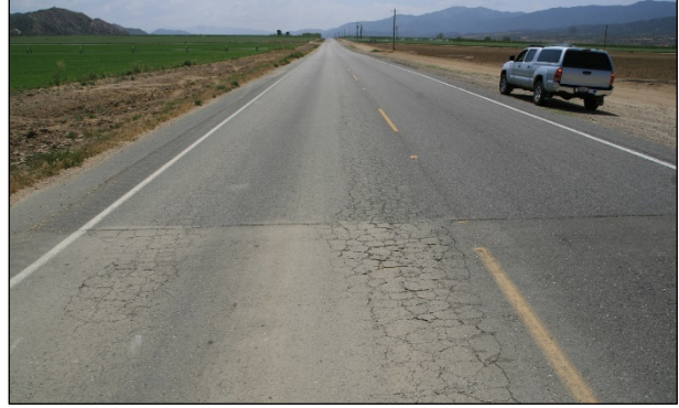
Figure 2.3: Example early full-width patch failure.
