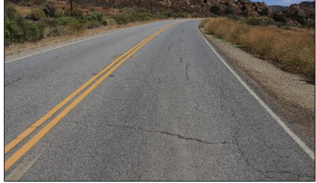
Figure 6.78: Early cracking caused by poor moisture distribution in recycled layer (FDR).
