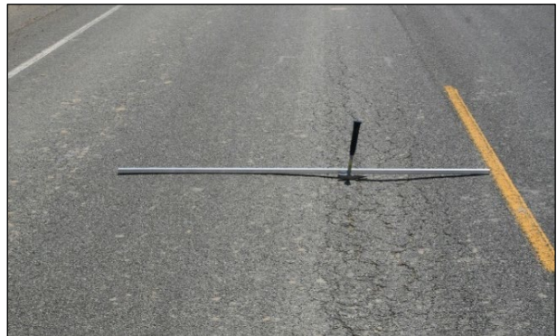
Figure 2.5: Example rutting associated with base/subgrade failure.
