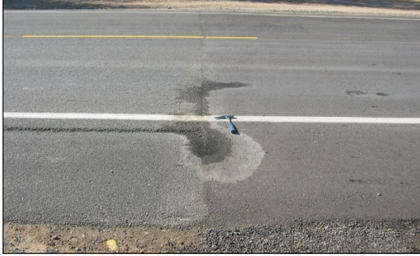
Figure 2.29: Early failure in patch (note water pumping in joint).
