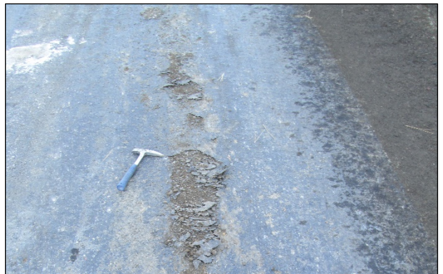
Figure 6.118: Delaminated area exposed during shrinkage crack mitigation (FDR-C).
