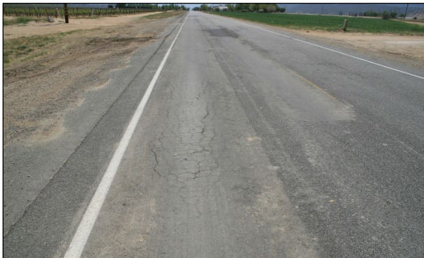
Figure 2.31: Early failure in wheelpath repairs.
