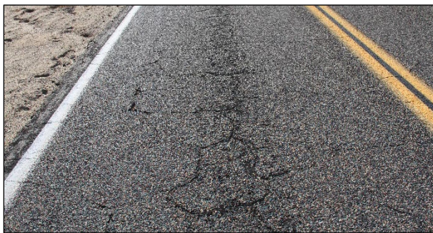
Figure 2.11: Example top-down distresses: Oxidative aging cracks.
