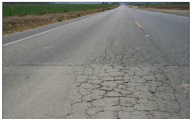
Figure 2.28: Early failure in patch (drainage problem).
