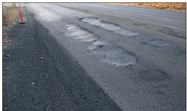
Figure 6.52: Trafficked recycled layer with severe raveling (patched) (PDR).
