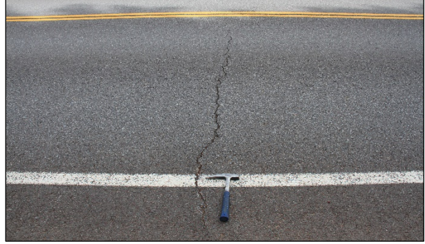
Figure 6.20: Early shrinkage cracks in area of accumulated cement (FDR-C).
