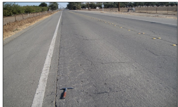
Figure 6.87: Fatigue cracking in asphalt concrete in the bridged area.
