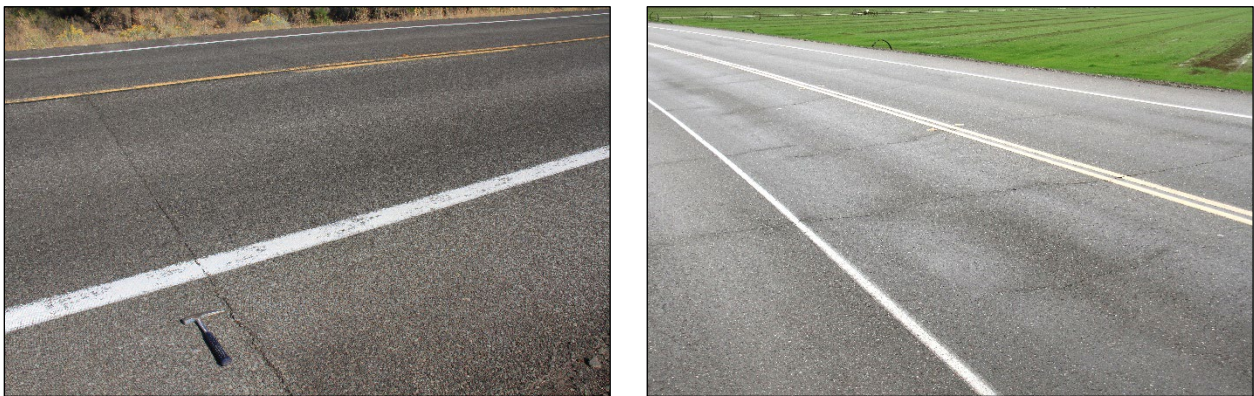
Figure 3.7: Reflected shrinkage cracks on FDR-C projects.
