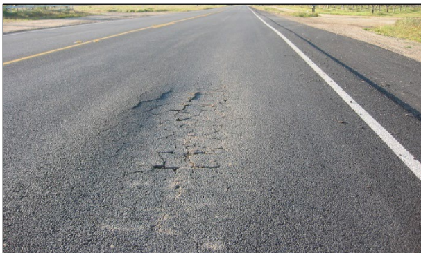
Figure 6.23: Localized early failure resulting from a wet area (FDR).
