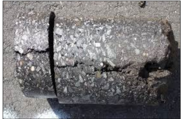
Figure 2.42: Bottom-up fatigue/reflected crack.
