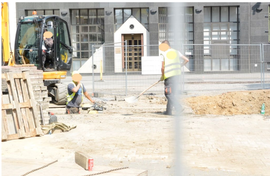
Figure 3. Roma construction workers digging a road in the center of Ostrava. Photo by author, May 2016.
